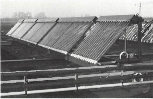
Fig. 18. Pilot installation with VTR141 tubes on the roof of the Philips central kitchens in Eindhoven.
